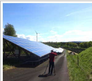
Solar arrays Photo: IfaS
